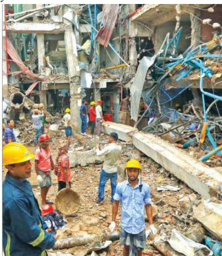
The remains of the building of Multi Fabs Limited after a boiler explosion. Photo: Prothom Alo, 7 July 2017.
